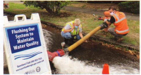
Crews continued flushing water mains in east Portland, cleaning out and maintaining water quality in close to 200 miles of water main.
